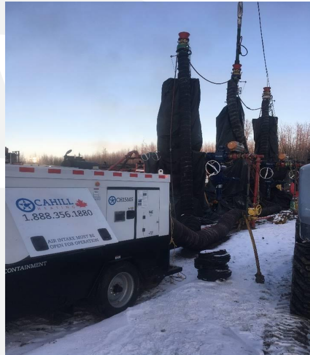
A CH15MS heater heating multiple BOPs simultaneously using split ducting on an oilfield
