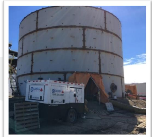
Delivering hot, dry, air to control humidity and temperature while coating a large tank
