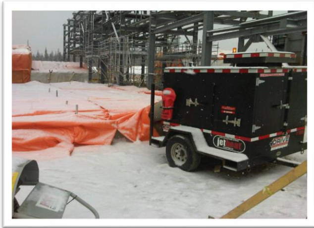
A CH15HS heater thawing out a large area of ground at a construction site in winter
